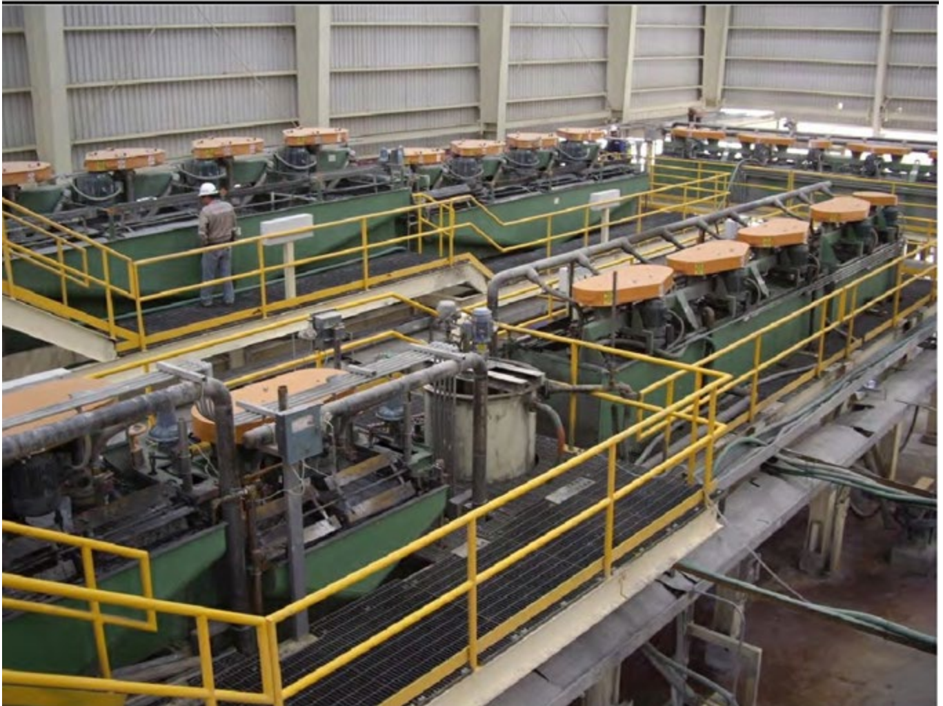
Figure 17-4: Banks of Flotation Cells at the DDGM Processing Facility
