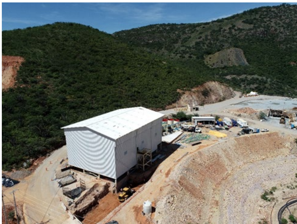
Figure 17-6: DDGM Tailings Filtration Plant
